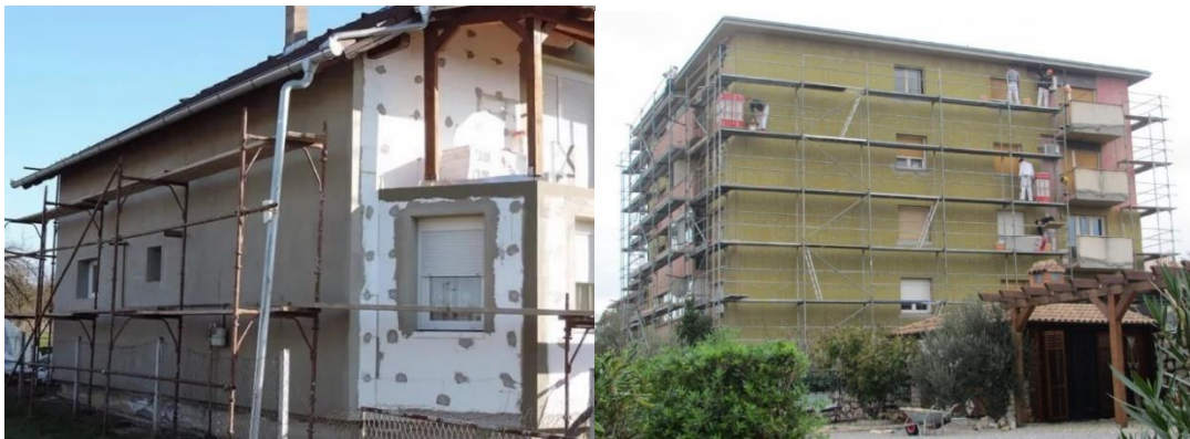
Fig. 1. Typical energy renovation construction sites - work on the external thermal envelope of family houses and apartment buildings[6, 7]
