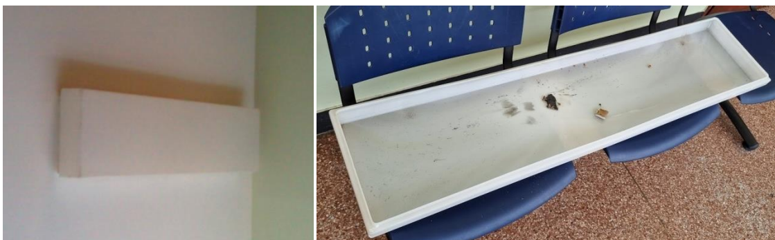
Fig. 6. The diffuser of the lighting fixture and pieces of the plastic housing of the ballast previously observed by thermographic inspection
