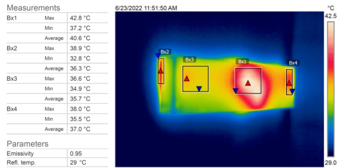
Fig. 3. Thermal pattern immediately after ballast failure
